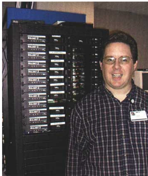
Bill Shewmaker with the newly installed Adtec Soloist 2 units
